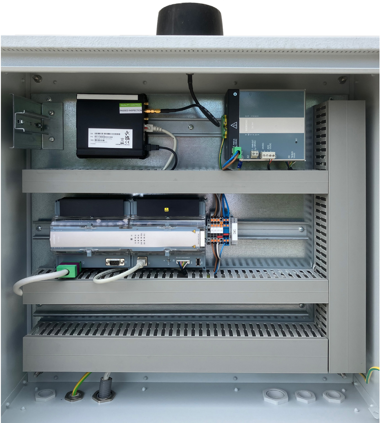
Antenna K7023231 used as End-Point Antenna in LTE450MHz Smart Meter Network.
